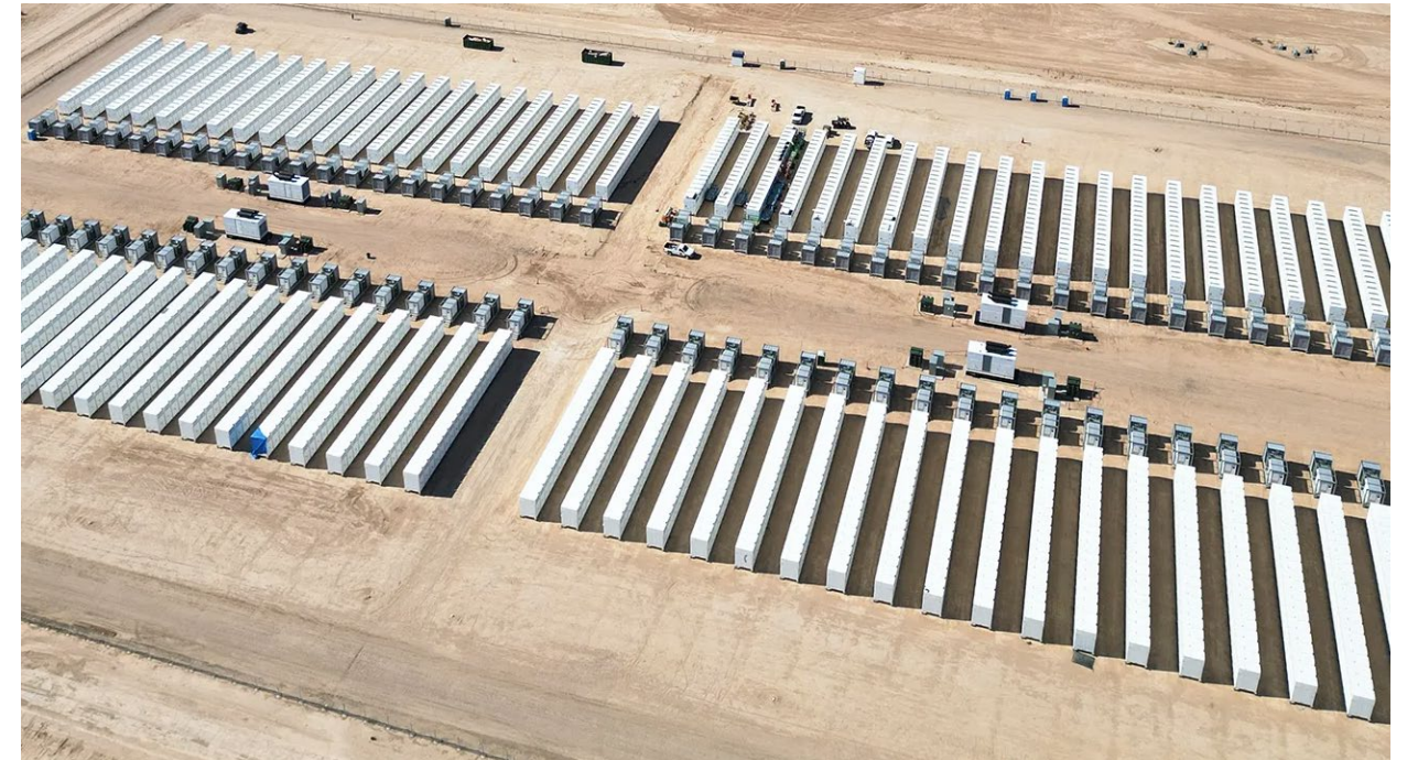
Sun Streams 3 Battery Yard
