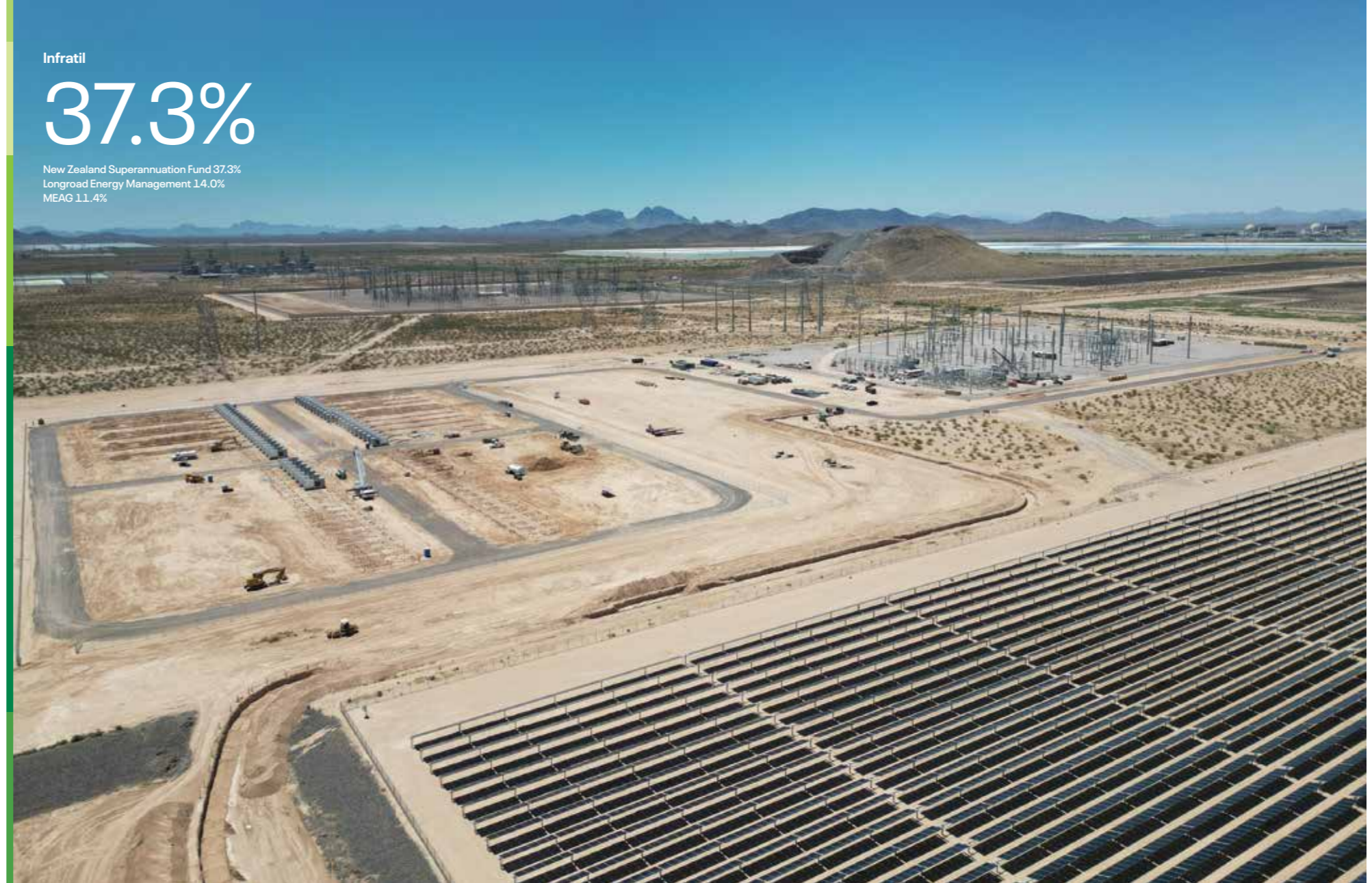
The switchyard and battery installation at the Sun Streams 4 solar farm, Arizona
