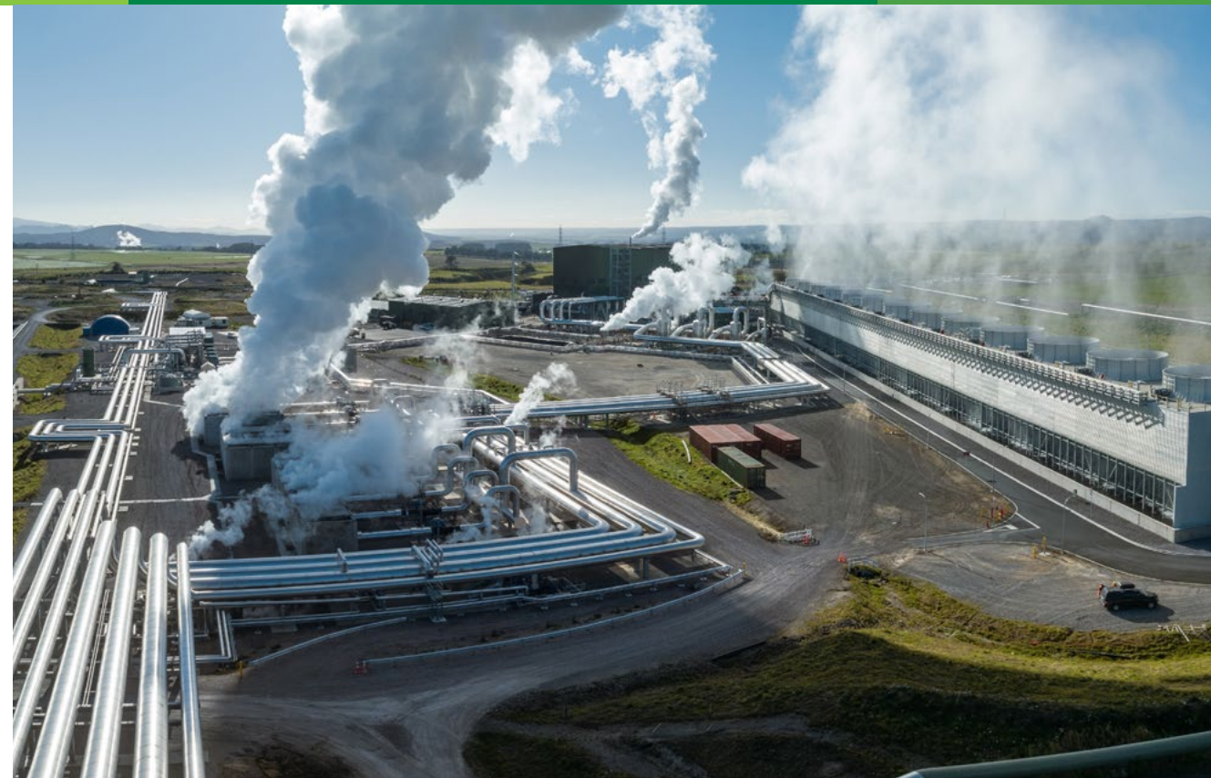
Contact's geothermal steam turbine power station at Tauhara, in Taupō, New Zealand.
