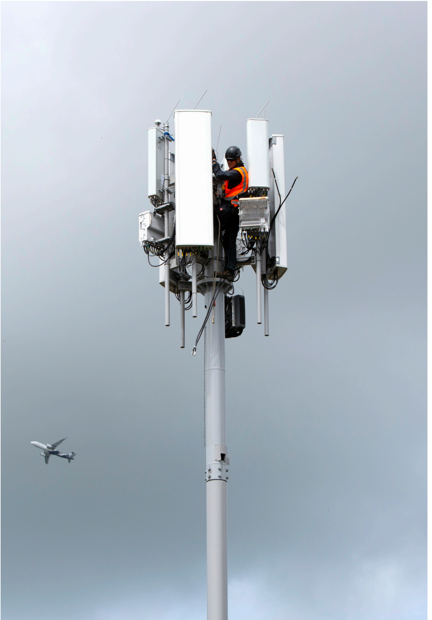
Vodafone 5G tower installation, Māngere, Auckland
