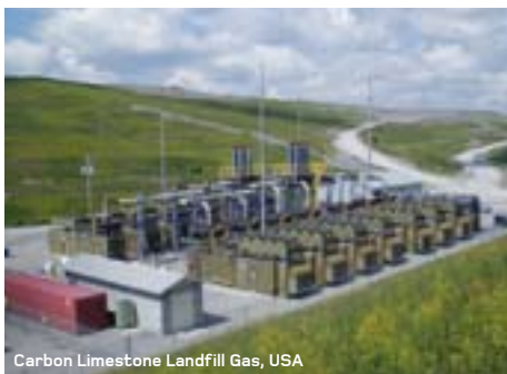
Carbon Limestone Landfill Gas, USA
