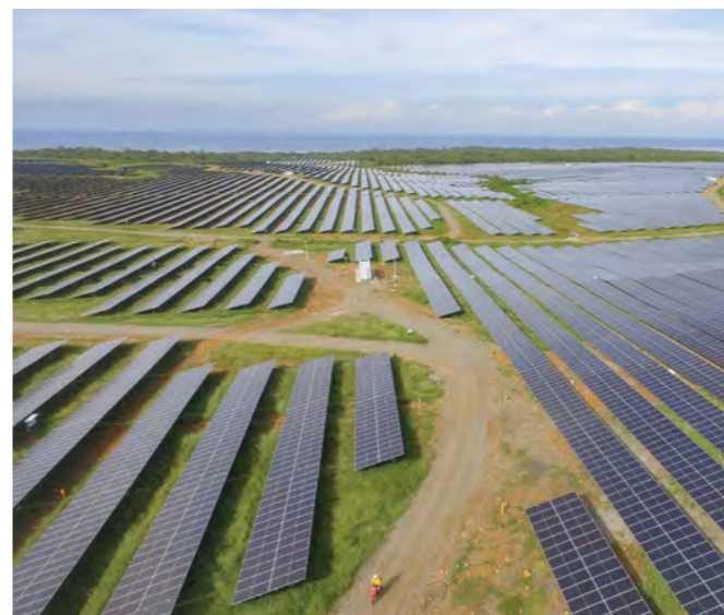
Gurin Energy's Palauig Solar Power Plant, Zambales Province, Philippines
