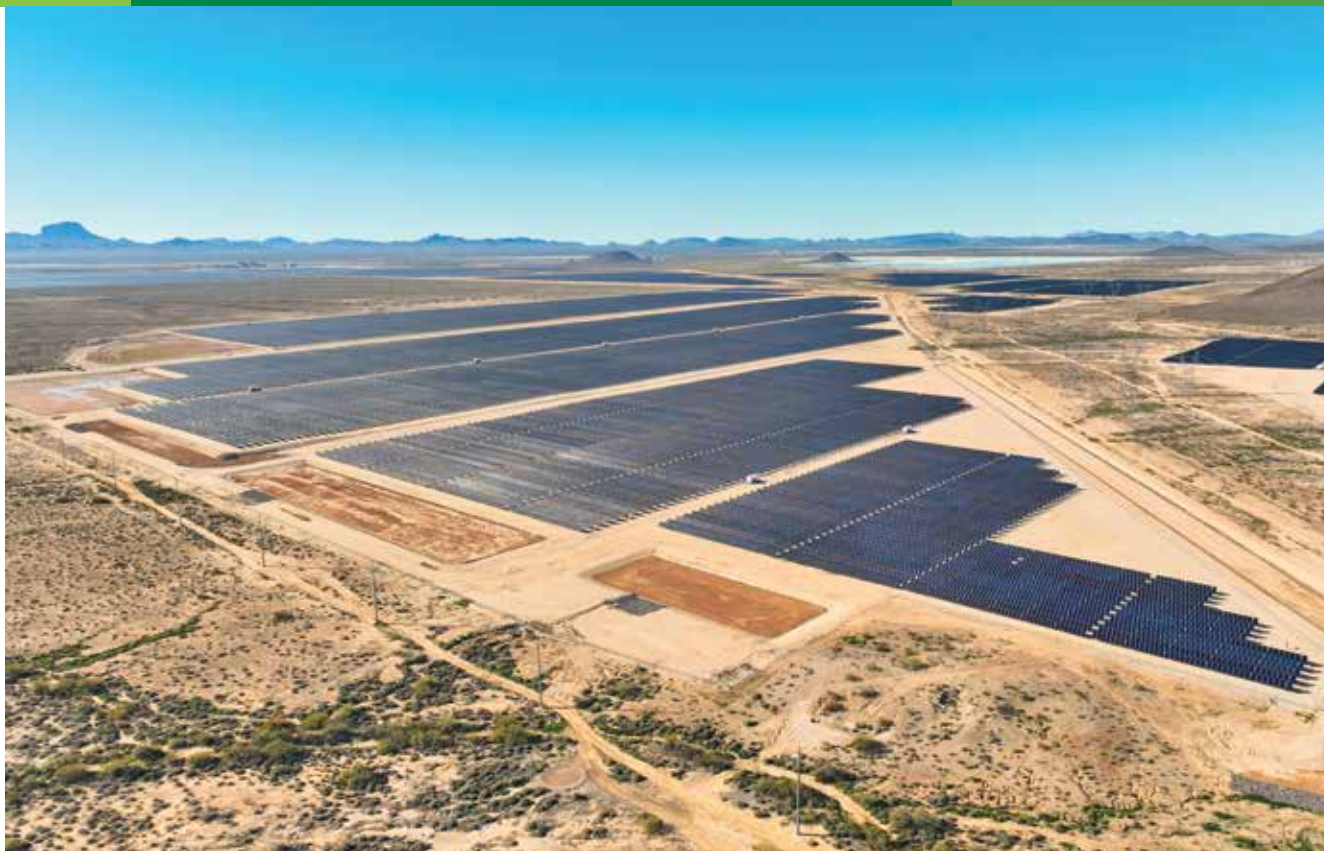
The Sun Pond solar and battery project in Arizona.
