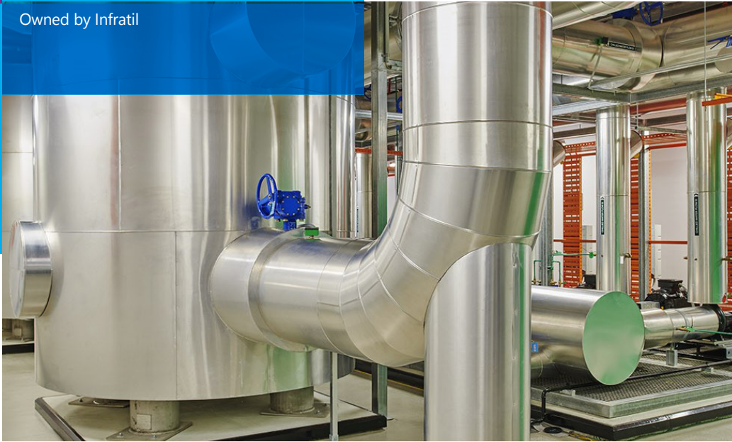
CDC's closed-looped cooling system.
